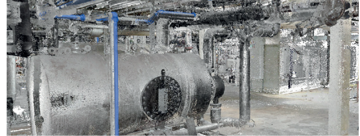
3D scan demonstrating how Polypipe can add value to your retro fit projects by scanning your building and overlaying with the exact MecFlow Fusion pipes and fittings you would need to complete your job.
